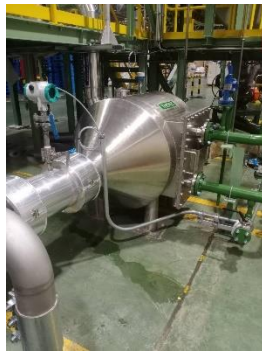
Water Cool Air Cooler
