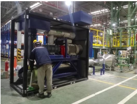
Roots Blower with Acoustic Enclosure
