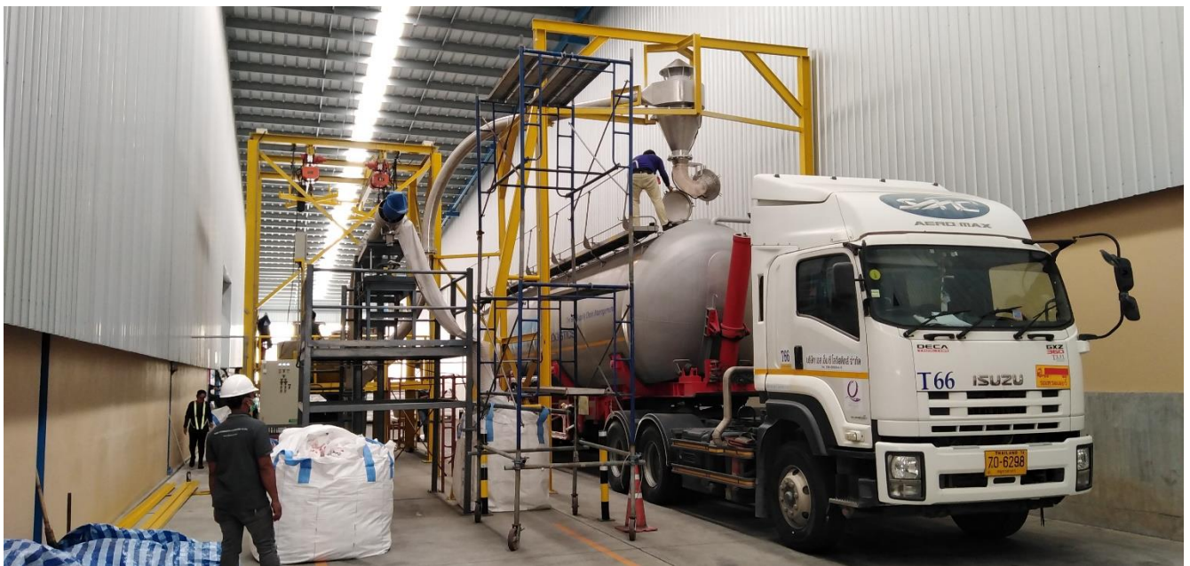
Installed in year 2020
